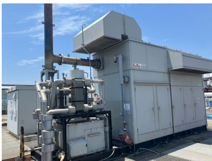
The 400kW gas engine cogeneration system, EP400G
