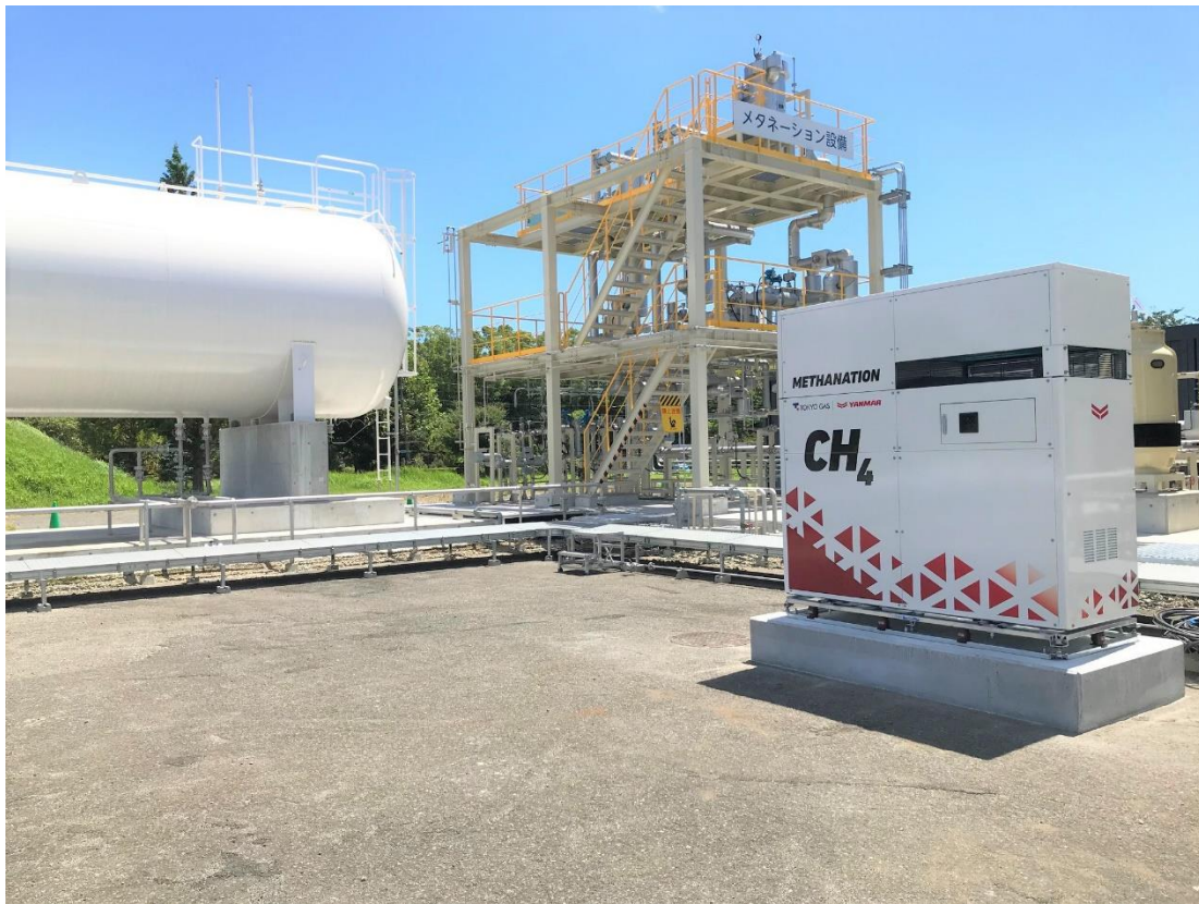
Cogeneration system (right) with methanation equipment (center).
